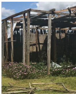
Cyclone Enawo inflicted significant damage to infrastructure.
